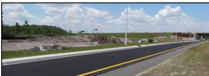
A new full interchange under construction on the Northern Coin System at SR 417 will provide better access between the two major roadways.
